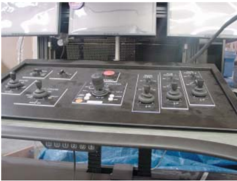
Crane operator’s control panel with six joysticks to be used in the Waste Treatment and Immobilization Plant (WTP) under construction at the U.S. Department of Energy’s Hanford, WA, site by Bechtel. Image courtesy of Washington Group.
